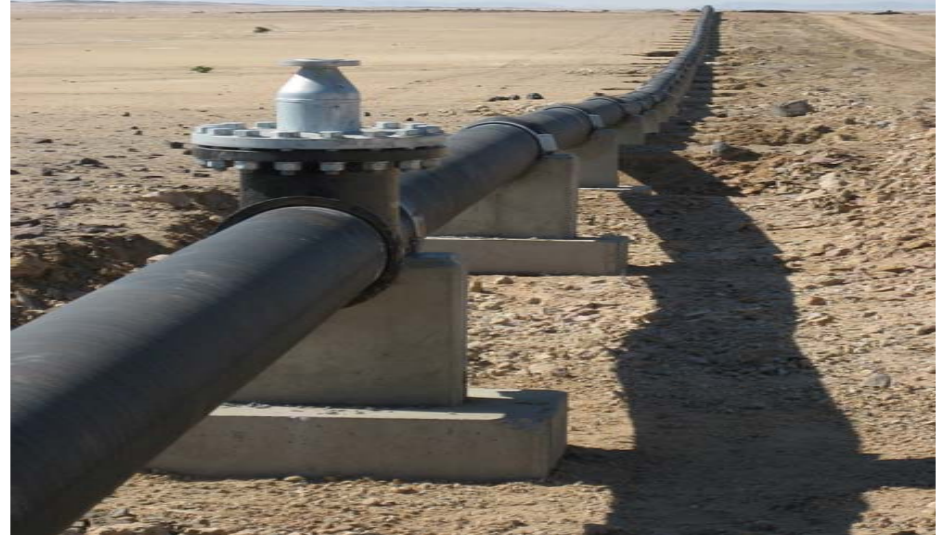
85km water pipeline (1.5m 3 pa)
